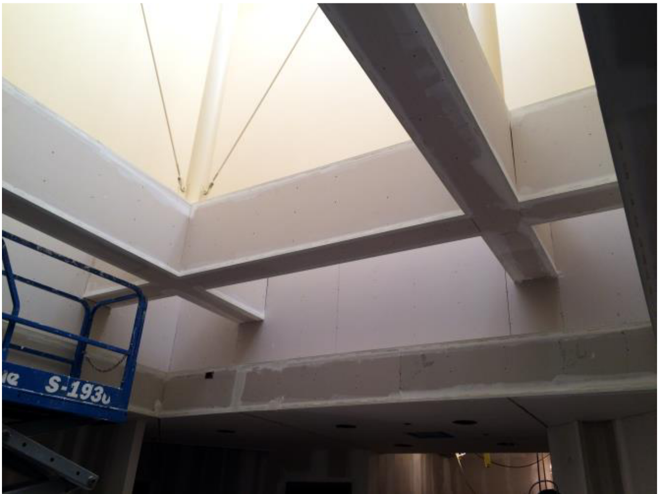
Soffits in the core (skylight) are complete. Finishing is underway. (Empire Lath and Plaster)
