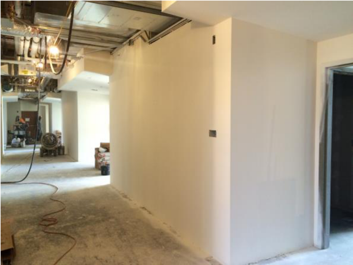
Floating is complete on the North side. Sanding is underway. (Empire Lath and Plaster)
