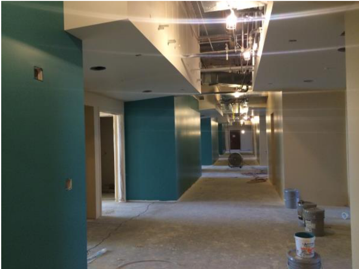
1 st coat of paint and accent walls in the West wing. (Excel Painting)
