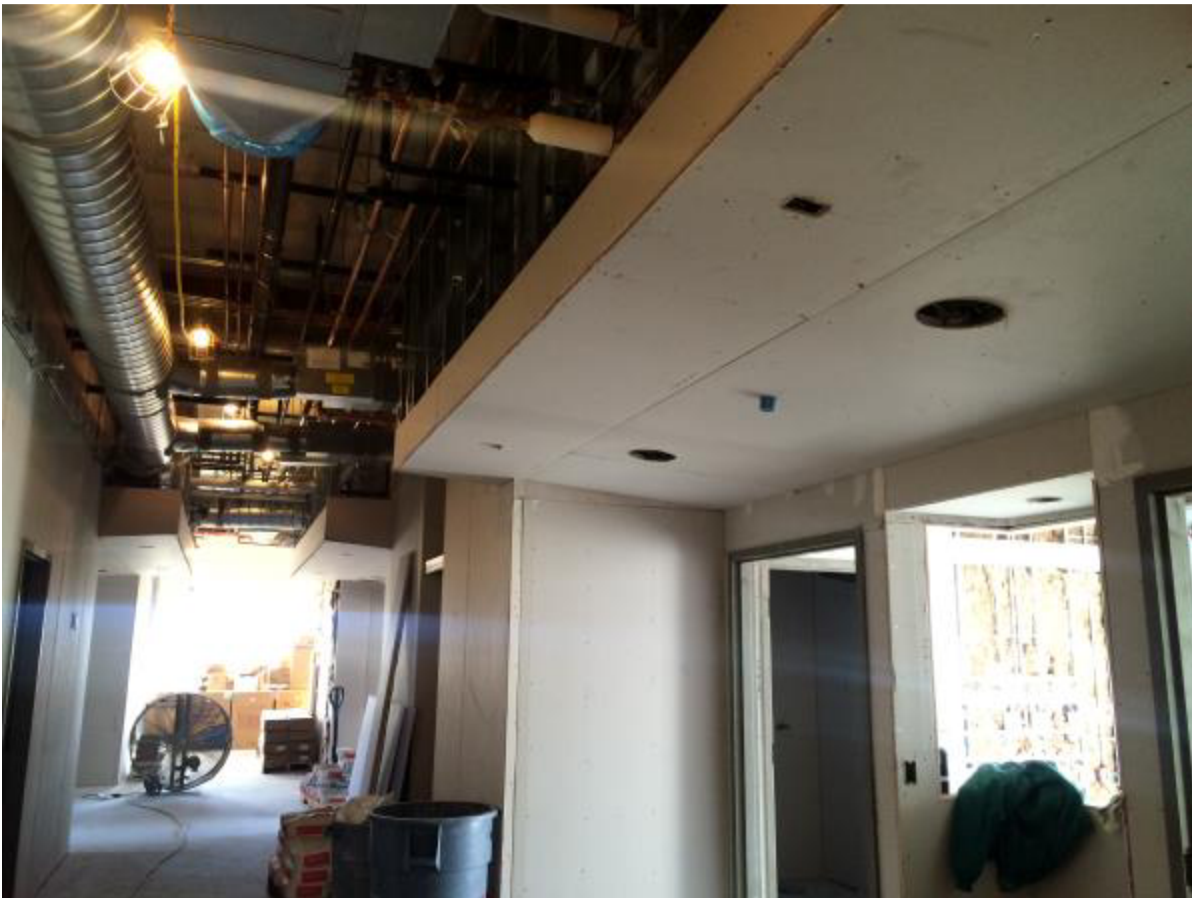
Soffits on the east side are complete with sheetrock. (Empire Lath and Plaster)
