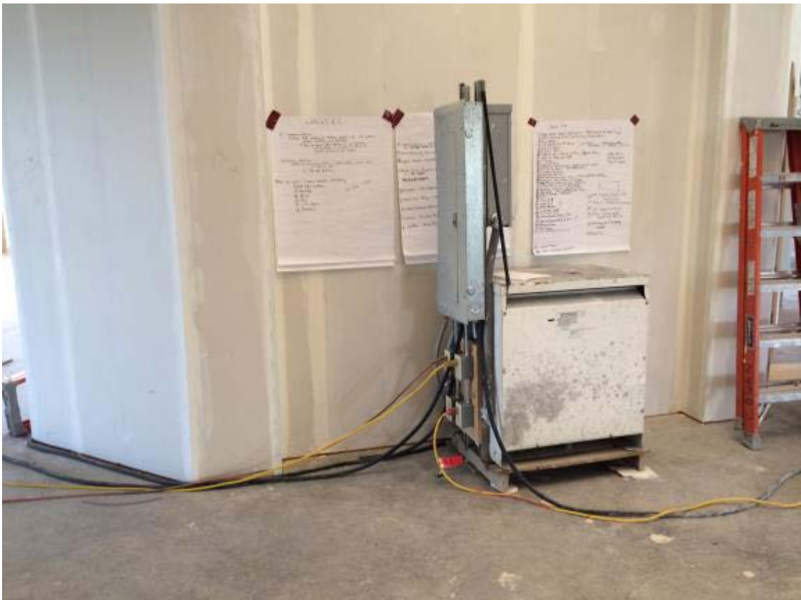
Temp Power is installed though out level 2 (Yellowstone Electric)
