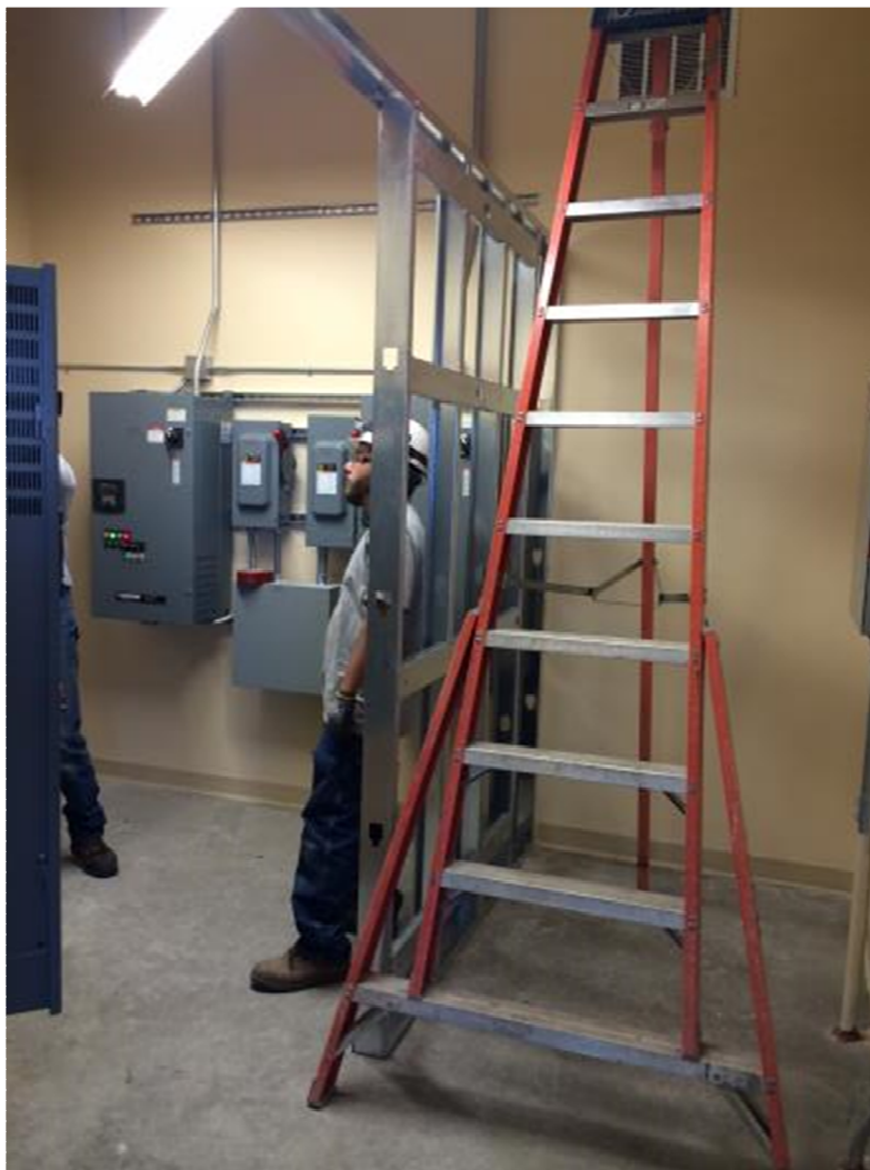
Electrical Room – New pony wall has been framed for new electrical gear. (Empire Lath and Plaster)
