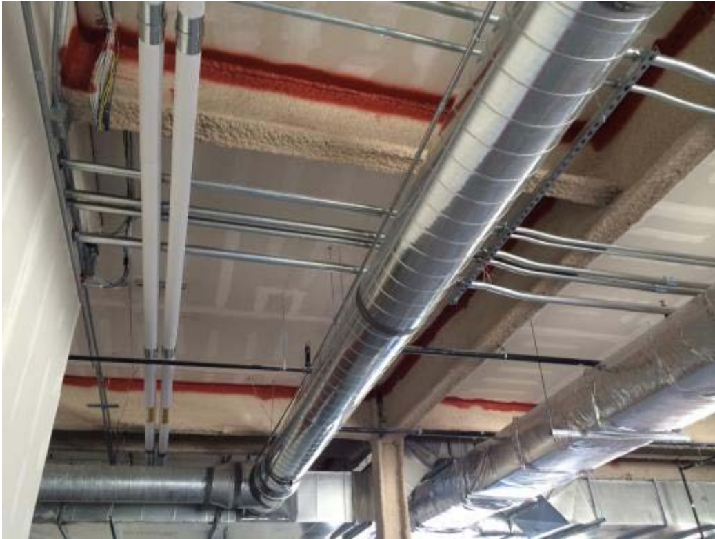
Main Electrical feeders (Yellowstone Electric)
