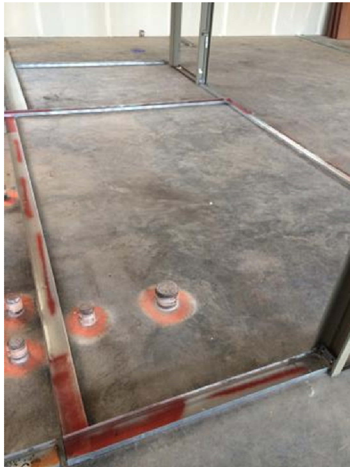
Layout and framing is underway on the west end. Red paint to identify rated walls. (Empire Lath and Plaster)
