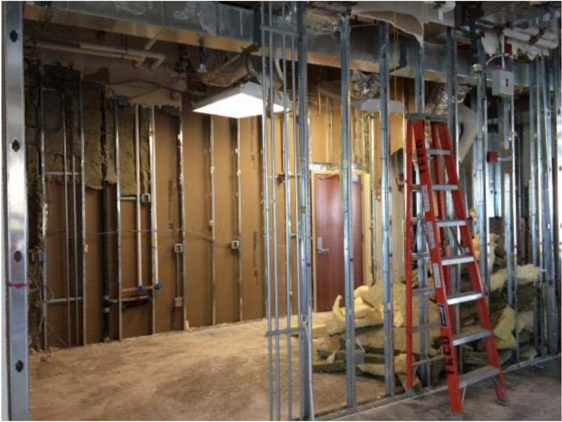
Demo work is underway on the "Family" room. Insulation is being saved for ICRA wall (Cowan Construction)
